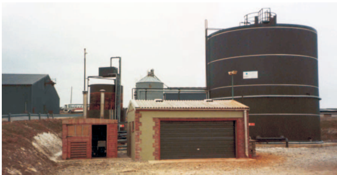
This 4 000 sow pig farm in South England using two gas engines (housed in the closed shed) to provide electricity for use on the farm as well as low grade heat for drying lucerne for horse feed as an ancillary farm operation.
