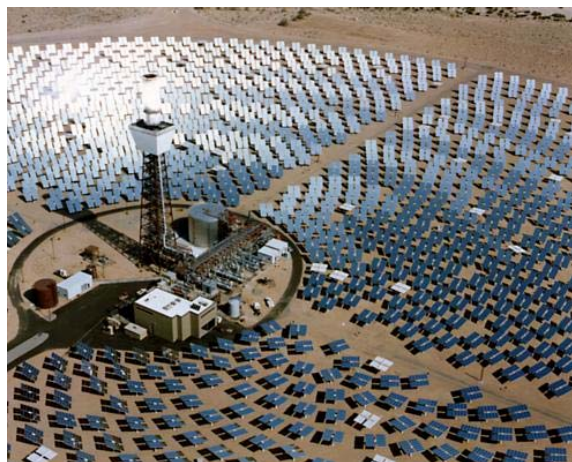
The Solar Two project in California USA uses a field of mirrors to focus solar energy onto a central boiler to produce steam and electricity. (Photo courtesy NREL).
